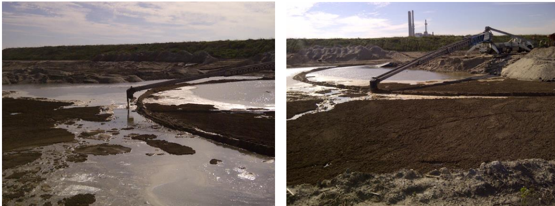
Figure 5. Site #4 USACE Chicago District John Mannville, Waukegan, IL Coal Ash Failure
